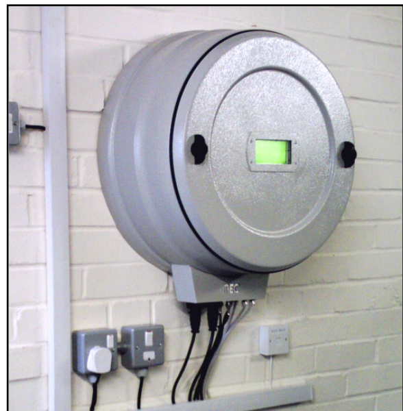
Figure 1: ASM On-line partial discharge monitor Data is sampled from each circuit at 100MSamples/sec, every 30 minutes giving a sufficiently high data resolution to accurately track variation in PD wave shapes, magnitudes and repetition rates over time.
